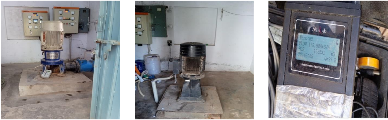
Figure 5: Sample pictures from field audit of pumpsets
